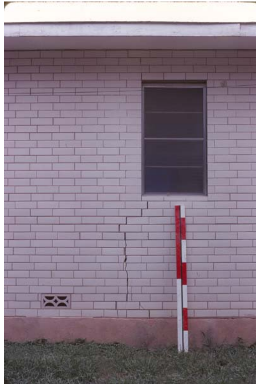
Figure 4-7. Structural Damage Attributed to Clay Substrate
