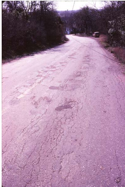
Figure 4-46. Road Destruction over Expansive Clay Substrate
