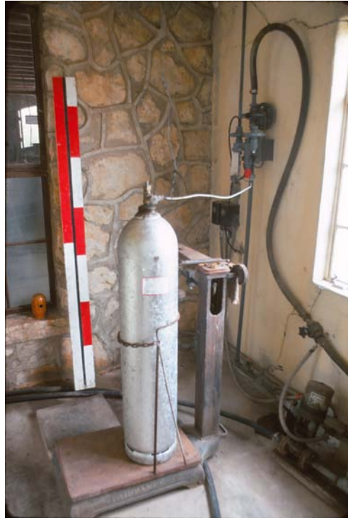
Figure 4-23. Water Treatment System for the City of San Marcos
