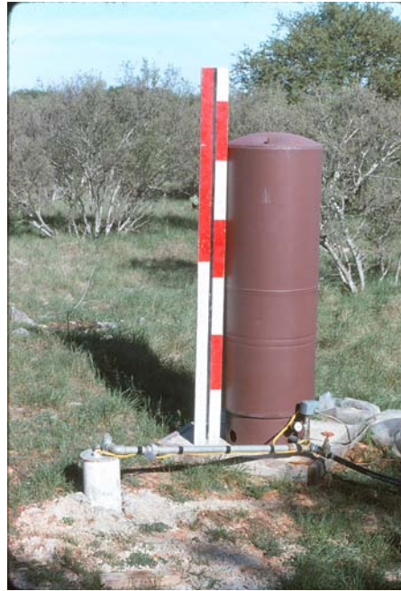
Figure 4-25. Typical Water Well Installed in the Outlying Developments
