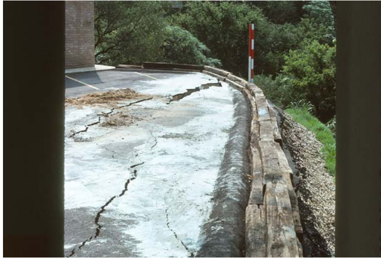
Figure 4-11. Slope Failure in Del Rio Clay Spoil Material
