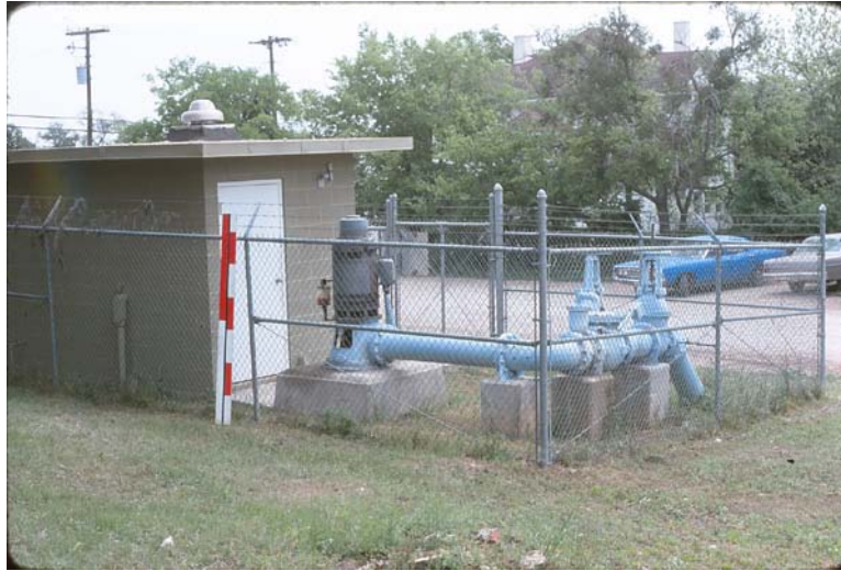
Figure 4-22. Municipal Water Wells
