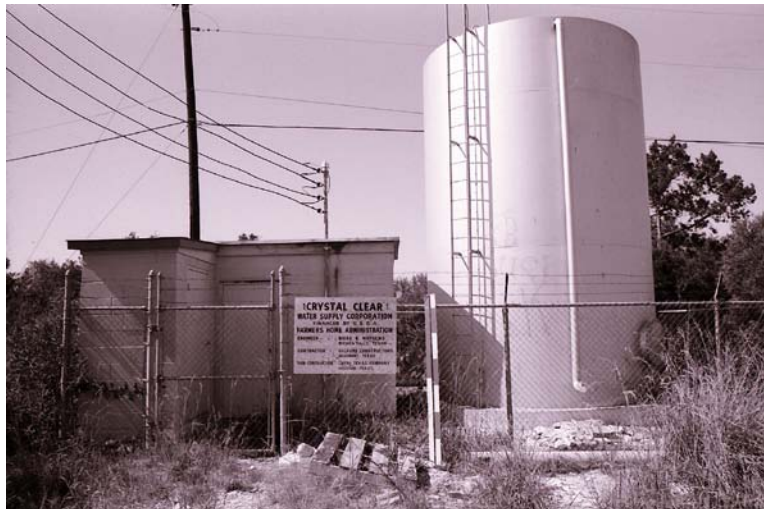
Figure 4-24. Pumphouse and Water Tank for a Water Well Operated by a Private Company
