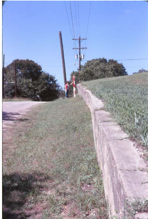
Figure 4-8. Failure of a Retaining Wall
