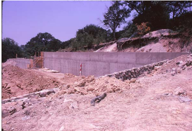
Figure 4-10. Slope Failure in the Del Rio Clay at an Apartment Complex
