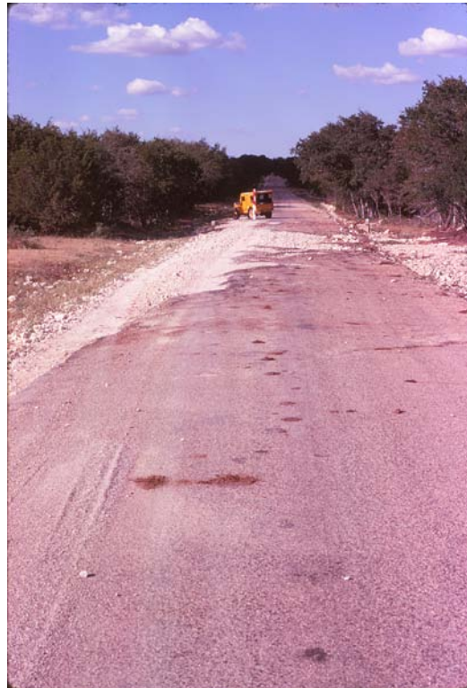
Figure 4-45. Road with Pavement Washed Out by Flooding
