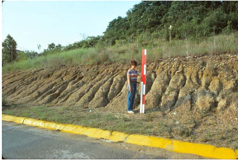
Figure 4-13. Rill Erosion of an Exposed Clay Slope
