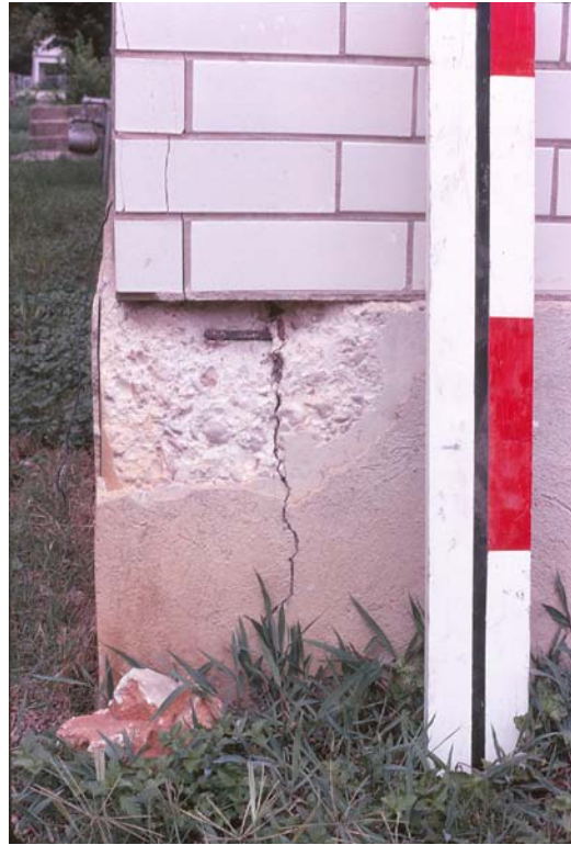
Figure 4-7. Structural Damage Attributed to Clay Substrate
