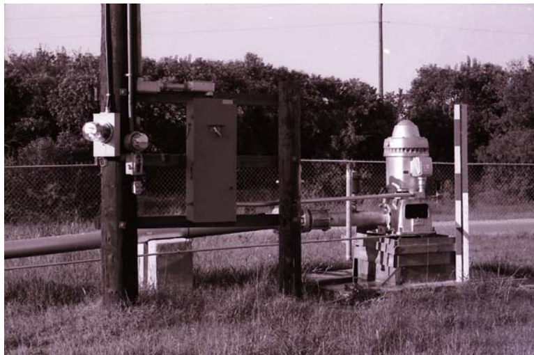
Figure 4-22. Municipal Water Wells
